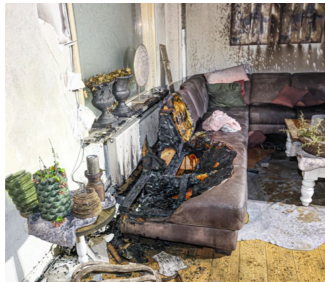
Middelbrand, bankstel in brand in woning Slagharen.
